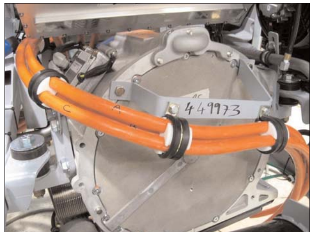
High voltage cables in orange coloured loom
