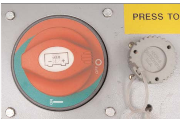
Master Disconnect Switch
