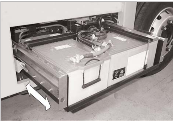
Vehicle 24 VDC Batteries (LHD vehicle shown)
