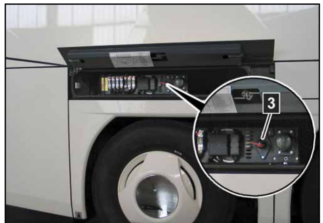
3 Battery isolator switch, coach (example, Cityliner)
