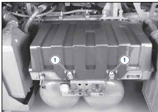
Battery box (batteries next to one another)
